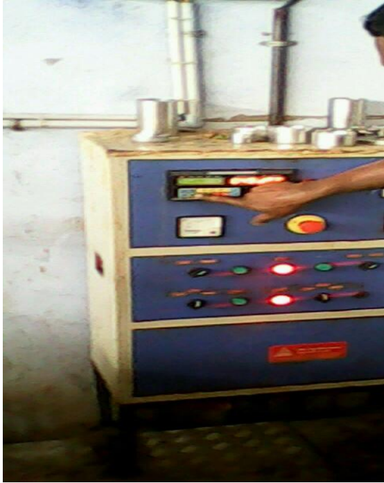
Setting the programme in main panel
