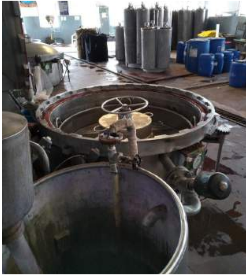
Photo: Addition tank, dyeing vessel and top carriers
